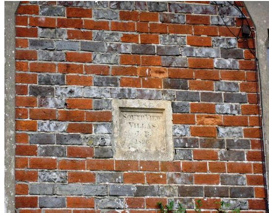
Glazed and unglazed patterned brickwork. South View Villas. 1896. Kintbury. Glazed and unglazed stretchers are grouped to form distinctive patterns.
