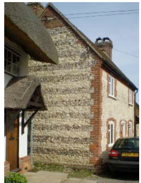
Berrick Salome: wall of banded flint and chalk clunch, with brick dressings
